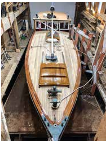
A new teak deck replaces the original canvas. Photo courtesy of T Burnett.
