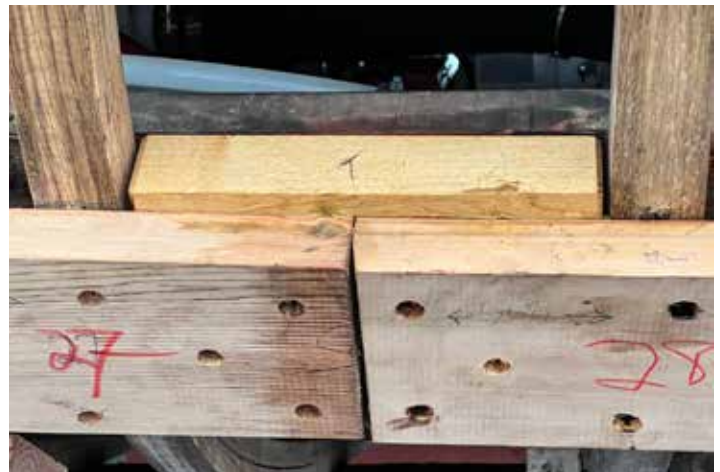
Illustration of new oak frames (verticals), locust butt block, and cedar planks. The board behind the butt block is an original fir stringer. photo by W Shain
