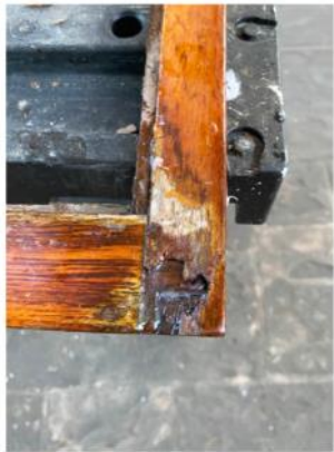
Near total failure of the window frame. Original wood glued up before fresh teak is applied.
