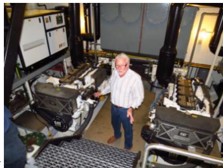
Dave Olson showing Acania's engine room
