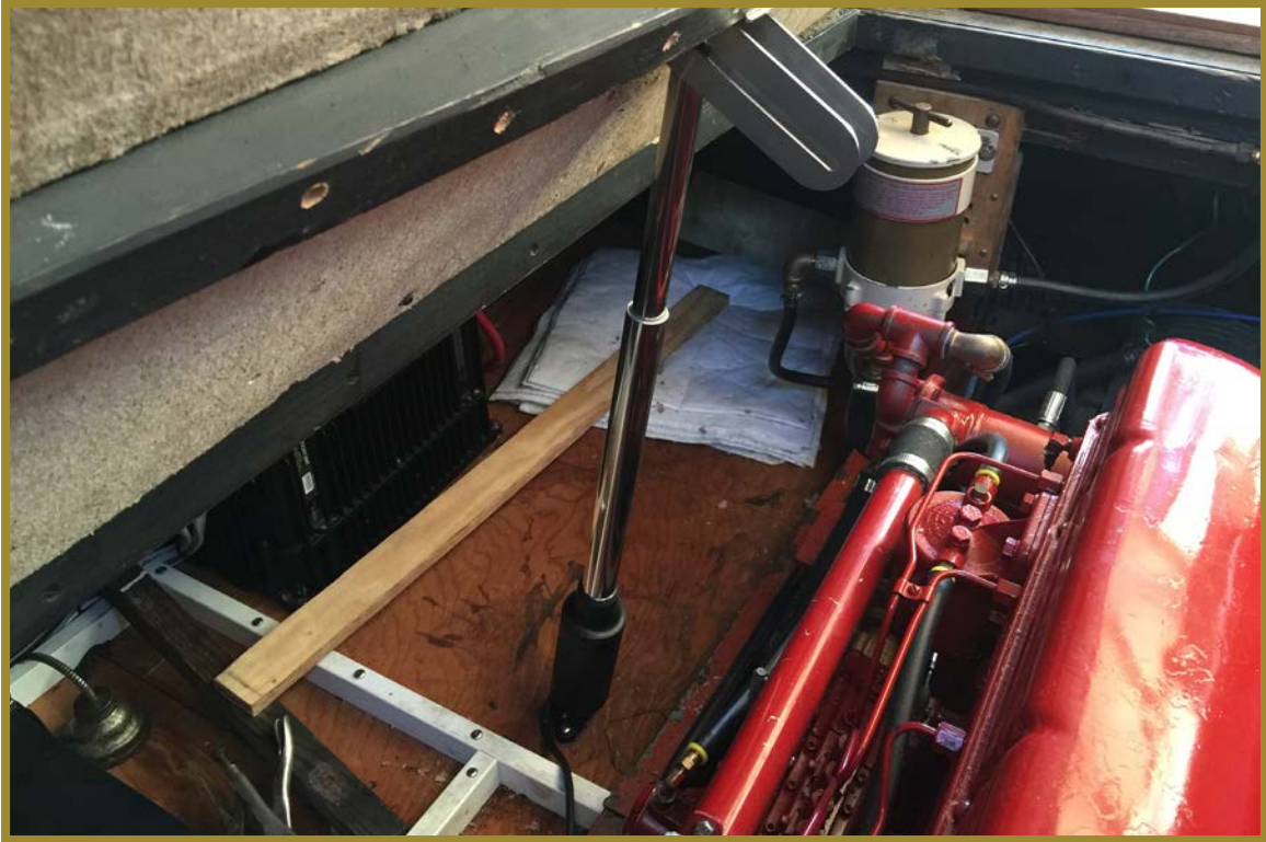
This lift was installed to help with opening and closing the heavy hatch
