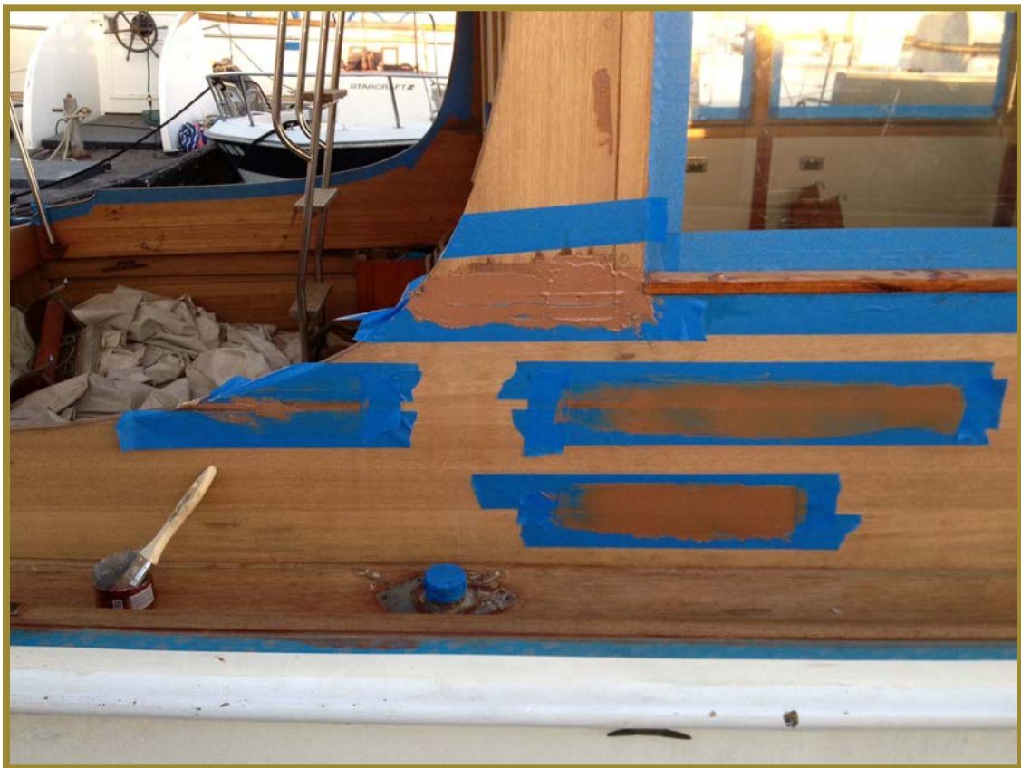
Along the way, we made many needed wood repairs on the Vera Lee's exterior.
