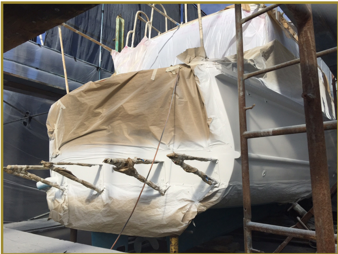
3 coats were applied to Vera Lee II's sides. A coat of high built epoxy primer, one coat of finish primer and a coat of Alexseal cloud white coating.
